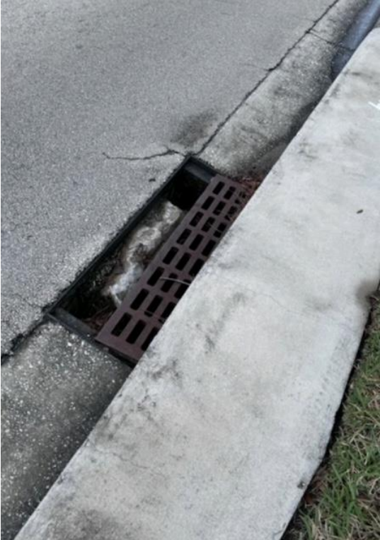
Solterra Blvd Grate – Before
