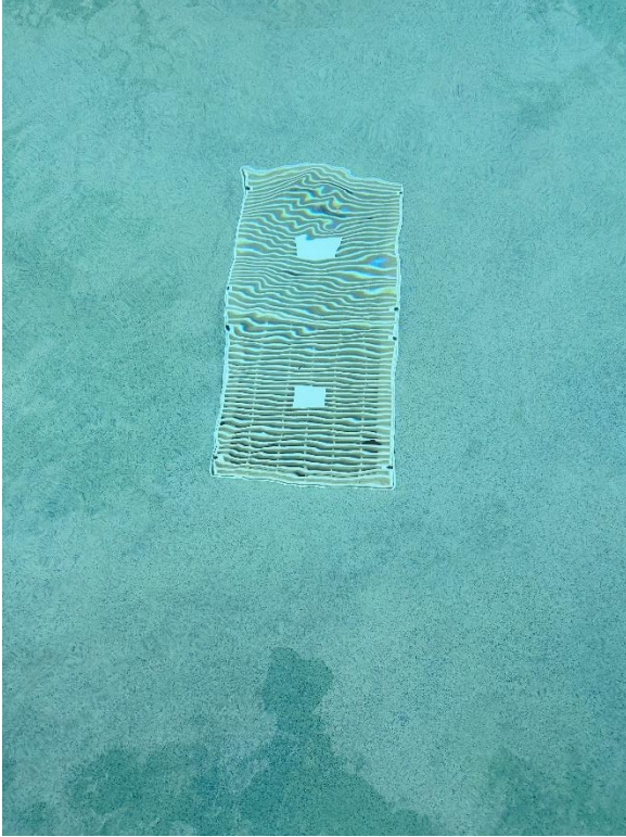
Pool Main Drain – Before
