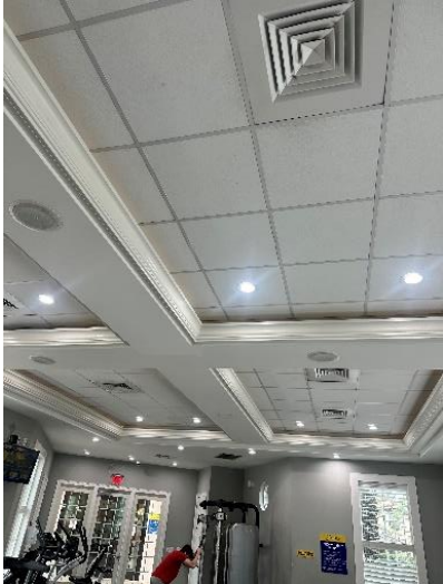
LED Conversion - GYM After
